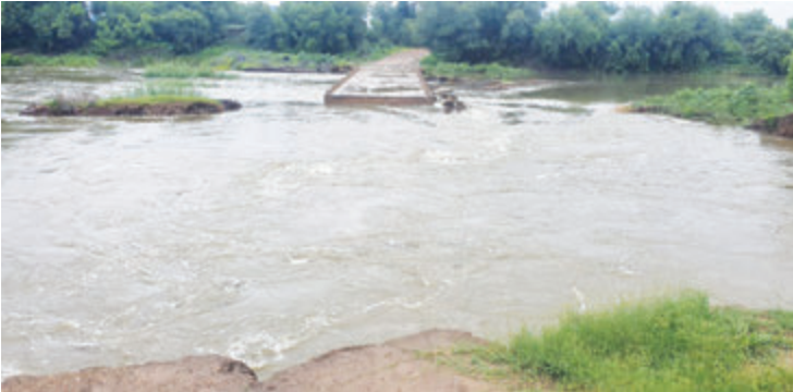
Motorist are urged to avoid this bridge. (photo taken from Northam Platinum Mine’s side).
